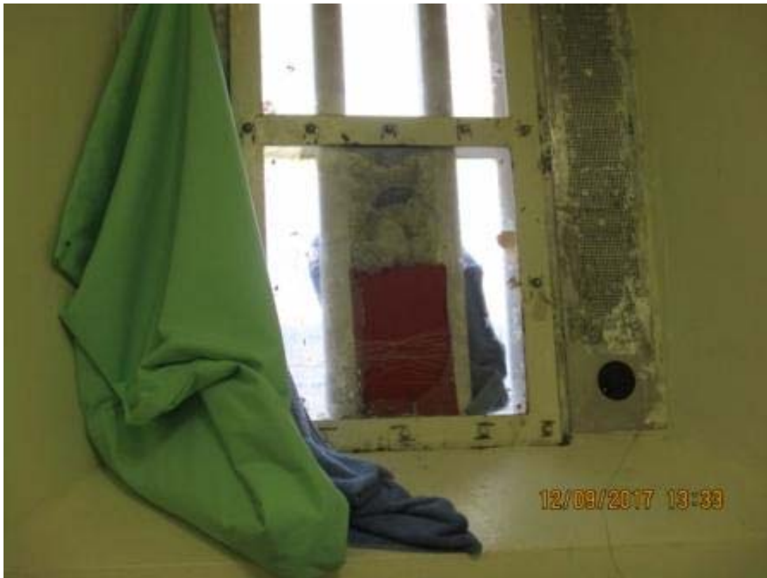
Broken window in a cell
