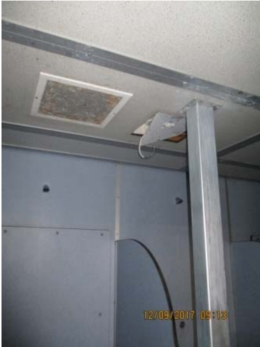
Shower unit with protruding electric cable
