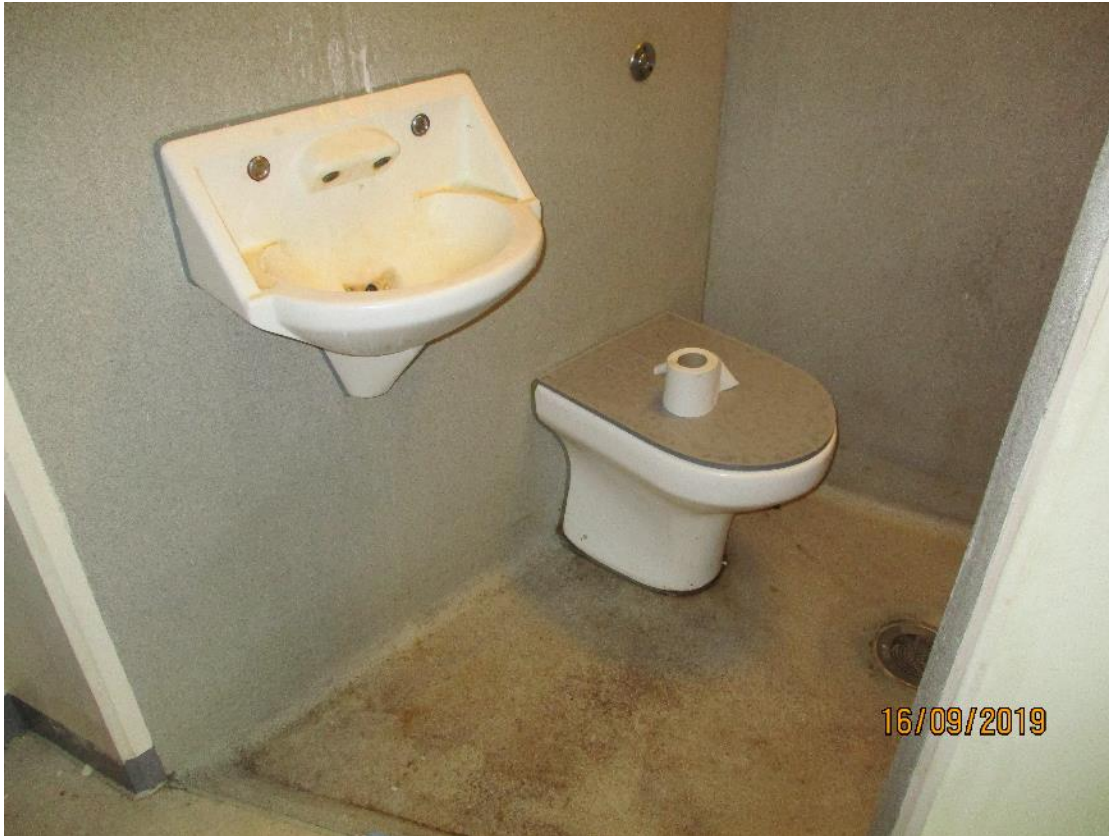
Dirty shower area
