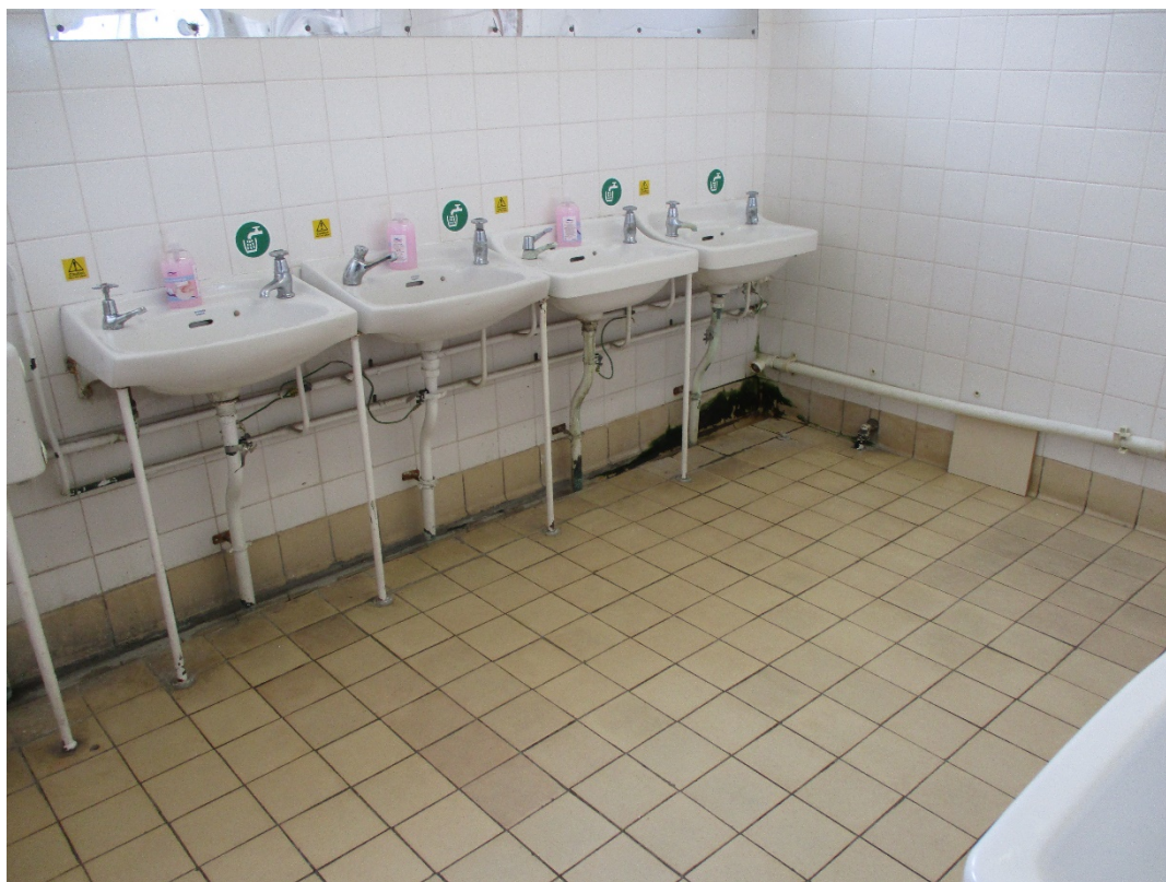
Mould on shower room floor
