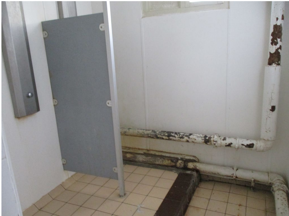
Condition of C wing showers
