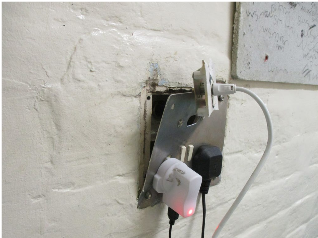
Loose electrical fitting
