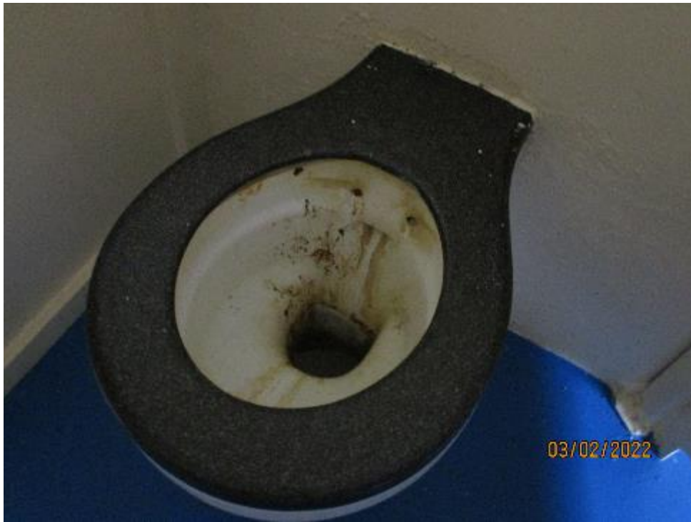
Badly stained toilet on Doulton unit
