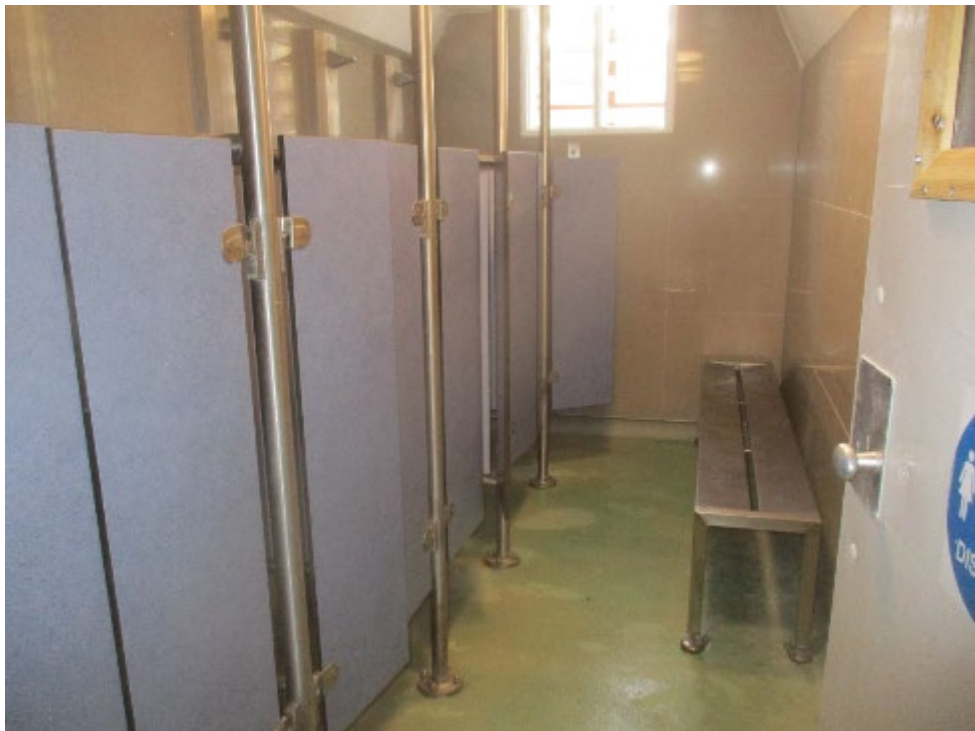
C wing showers during the 2021 inspection (top) and during this review of progress
