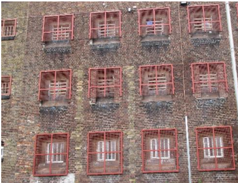
Rubbish in the window grilles during the 2021 inspection (top) and during this review of progress
