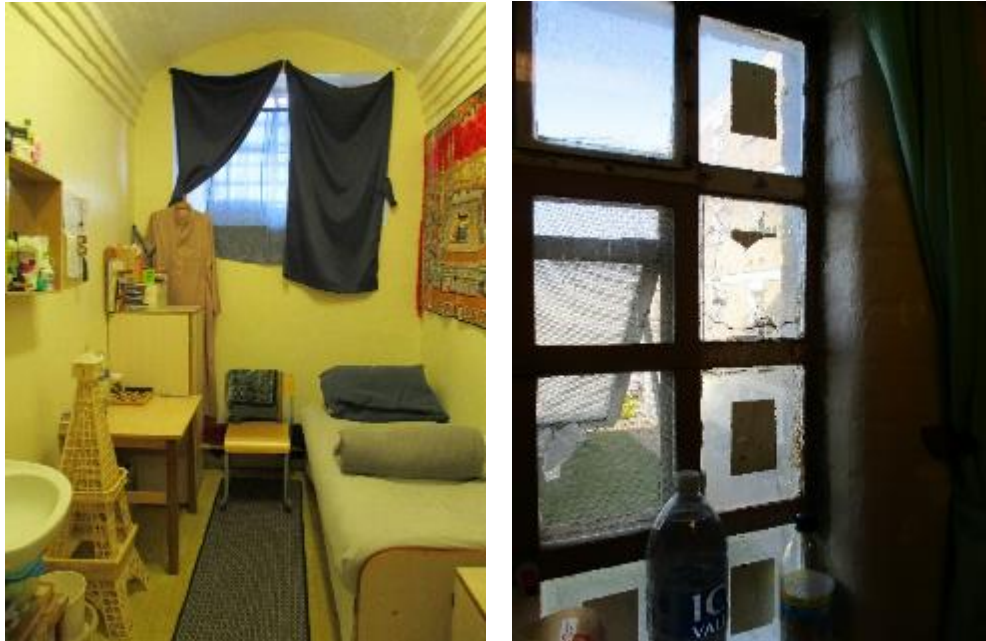
Personalised cell on Kent wing (left) and damaged window on Medway
