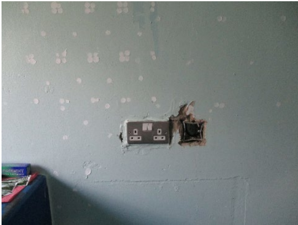
Damaged aerial point in a segregation cell
