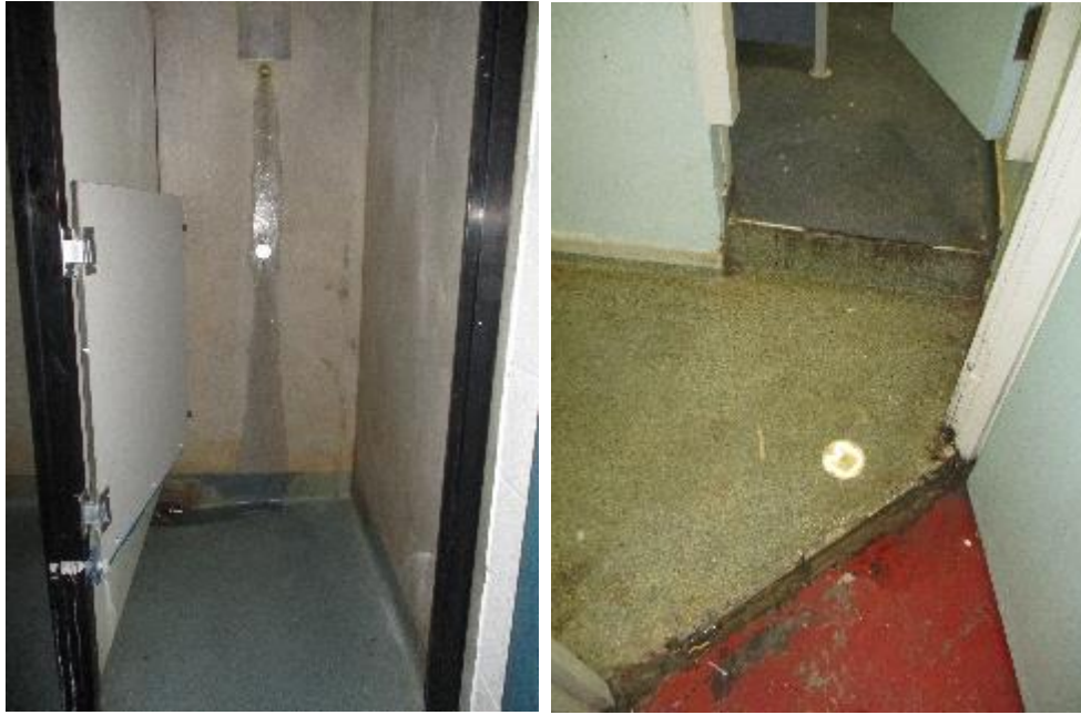
Shower unit (left) and inadequate drainage in a shower unit
