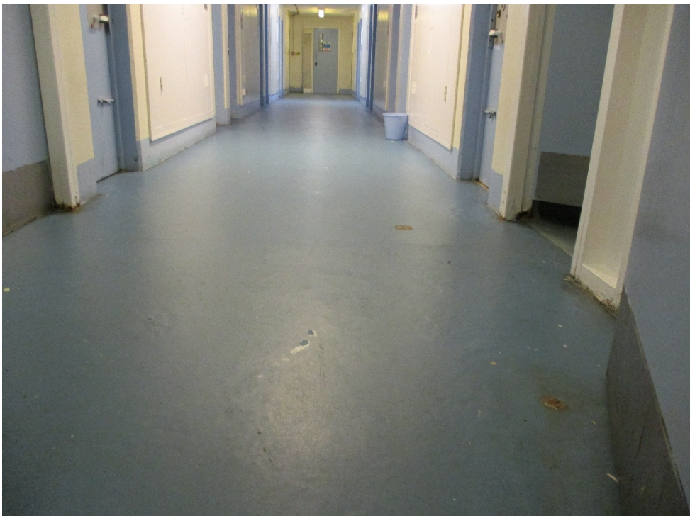
Poor flooring on A wing
